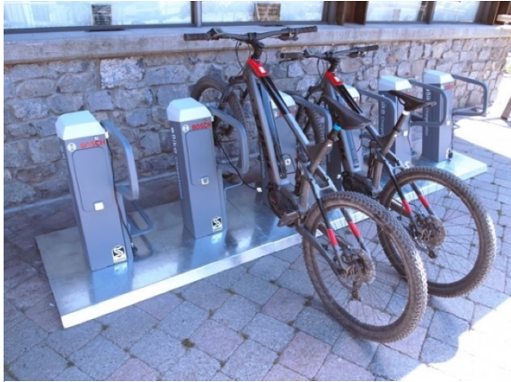
Figure 10. E-Bike Charging Stations
